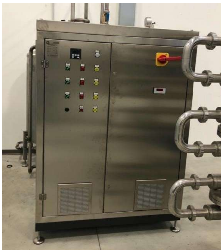
Figure 15 Heat Steam Generator
