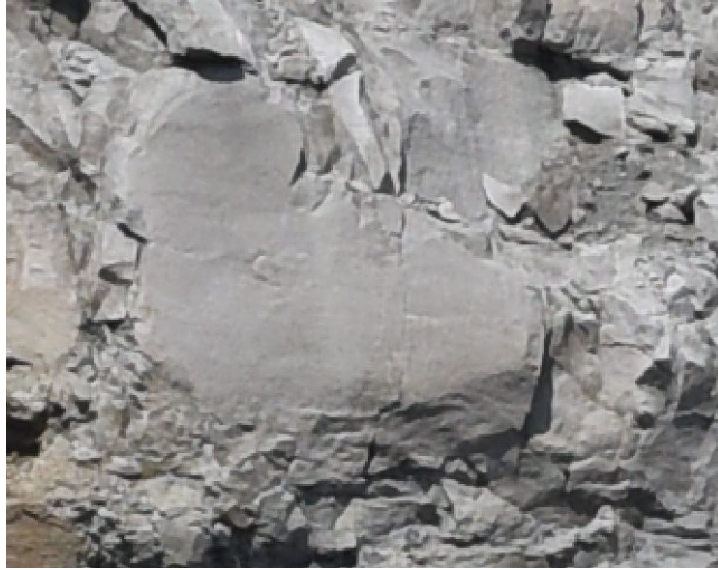
Figure 4-20: Flat untextured surface on the Glendale rock wall
