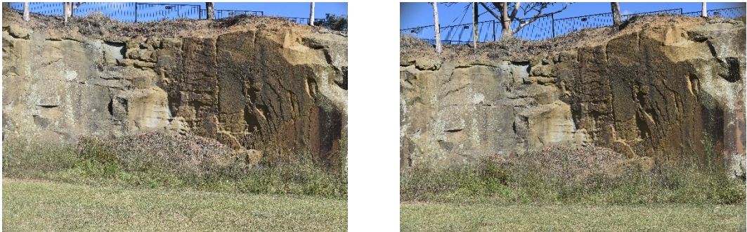
Figure 4-13: Pilkington rock wall image pair acquired with the stereo fixed photogrammetric system illustrated in section 4.1.3.
