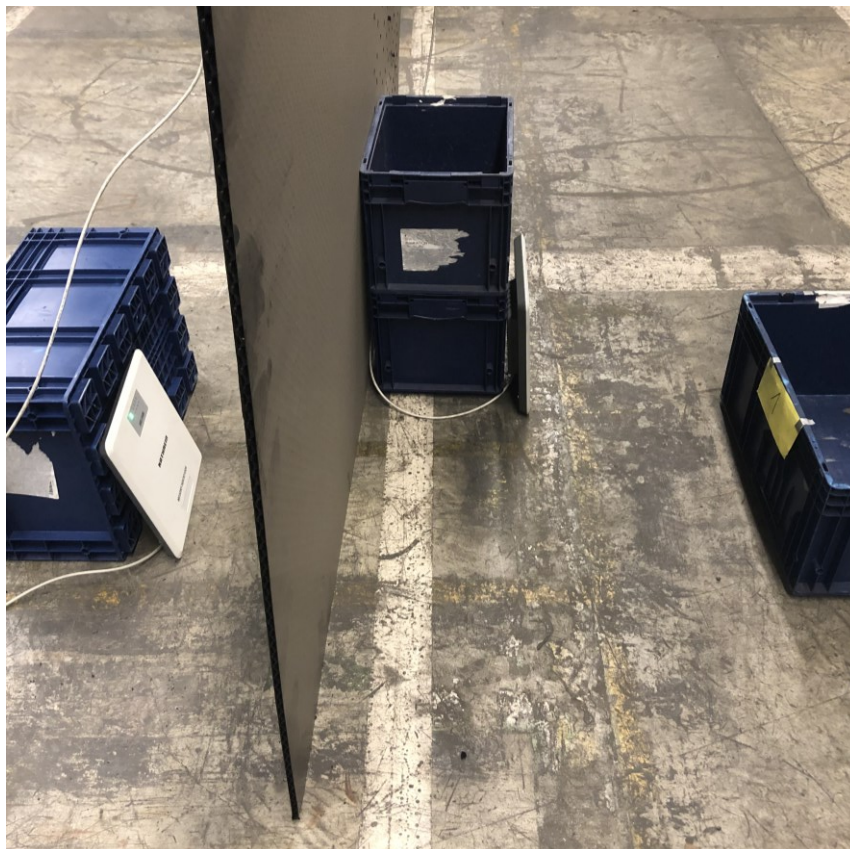
Figure 51 Setup of the RFID installation for the verification of the reader-to-transponder signal collision test
