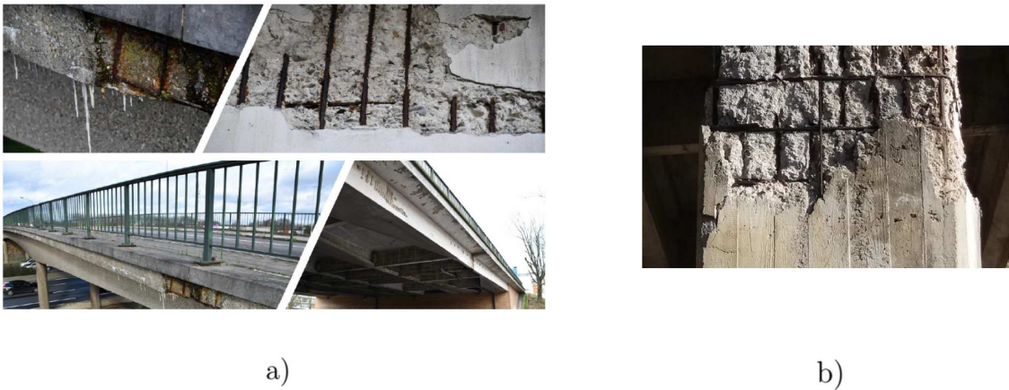
Figure 1.2: Example of corrosion of rebars in reinforced concrete structures. a) examples of concrete spalling from [14]; b) concrete cover spalling induced by corrosion of rebars from [15]
