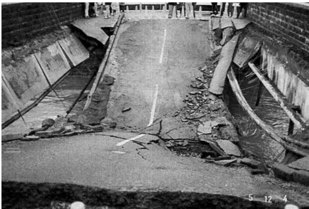
Figure 3-3 Collapse of the Ynys-y-Gwas Bridge, (Woodward & Williams, 1988). Reproduced with permission from ICE Publishing.
