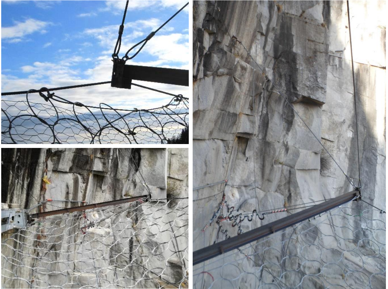
Figure 5.31: Barrier openings near post; a) Opening near post n. 2 before the test; b) Gaps near post n. 4 before the test and c) Gaps near post n. 4 after the test
