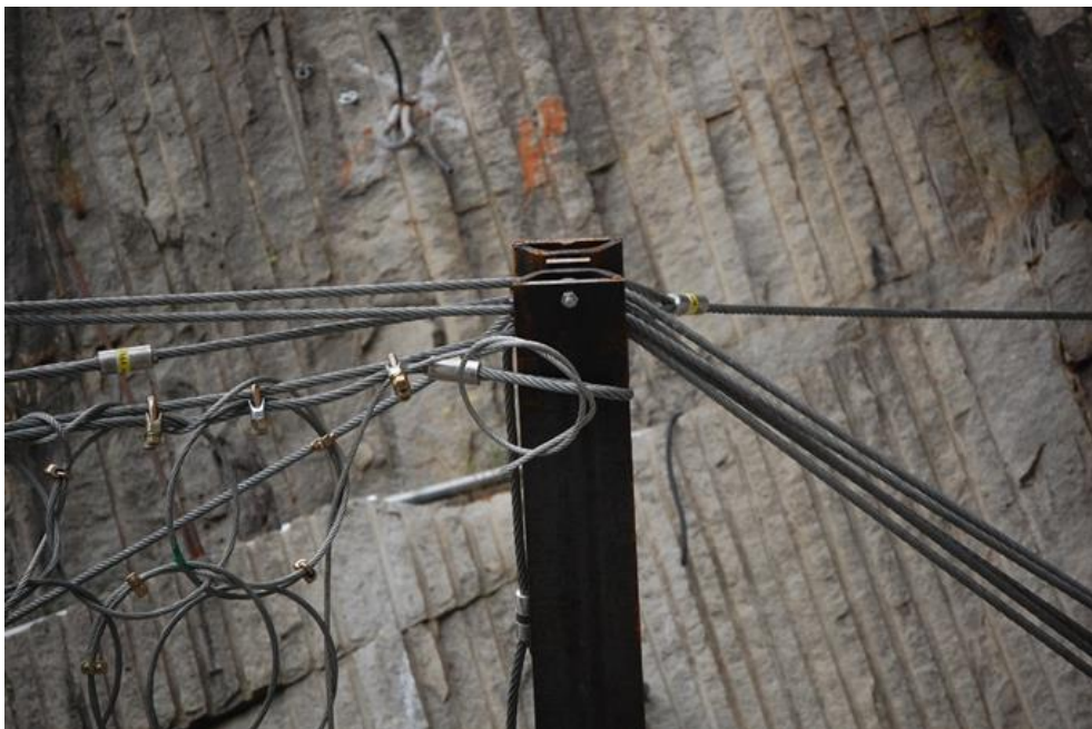
Figure 7.1: Post head detail, where the monitoring modules are positioned
