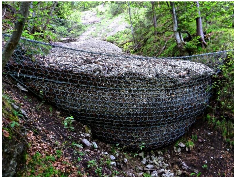
Figure 6.4: Example of a flexible barrier, horizontal cable and net under debris pressure
