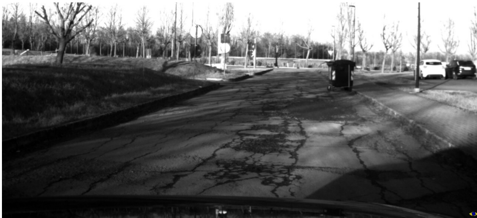
Figure 2.3: Missing lane markings on a old road.
