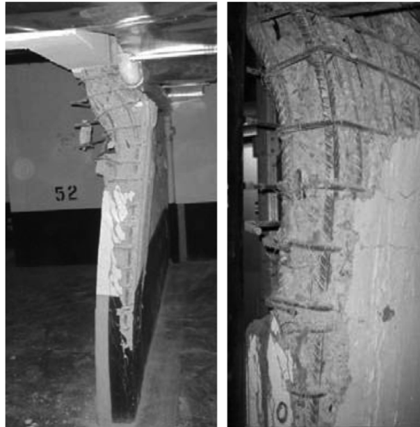
Figure 4.38 – Out-of-plane buckling of walls after 2010 Chile earthquake [Wallace, 2012].
