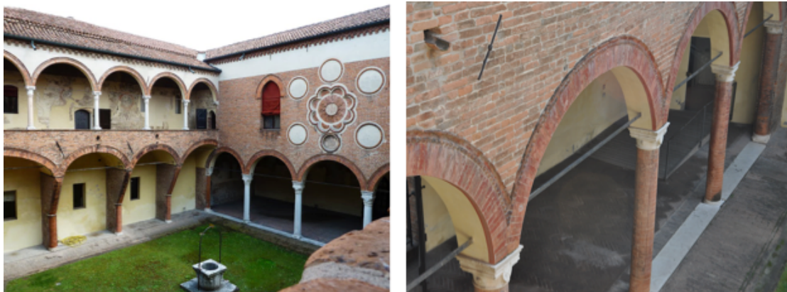
Figure 1.2. Inner yard of Casa Romei and zoom of the ground floor tie-rods.
