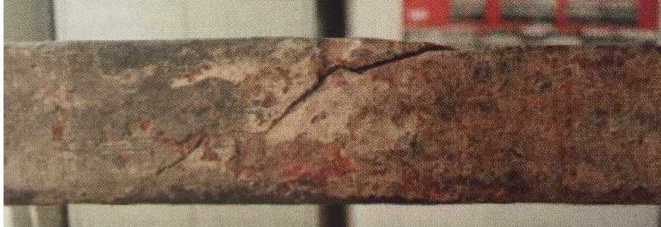
Figure 3.1. Crack in an ancient iron tie-rod
