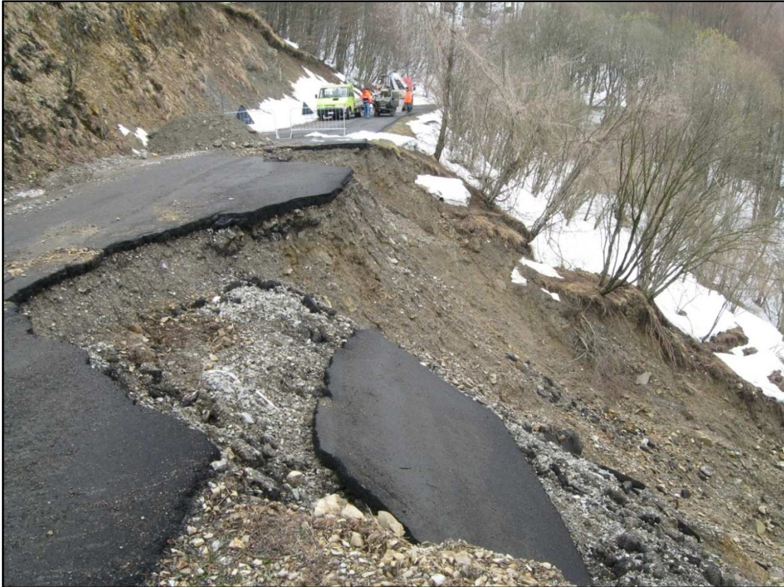
Figure 1.2 A road damaged by a superficial landslide (Tizzano Val Parma, April 2013)
